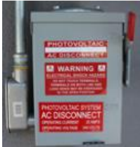
AC Disconnect Switch
