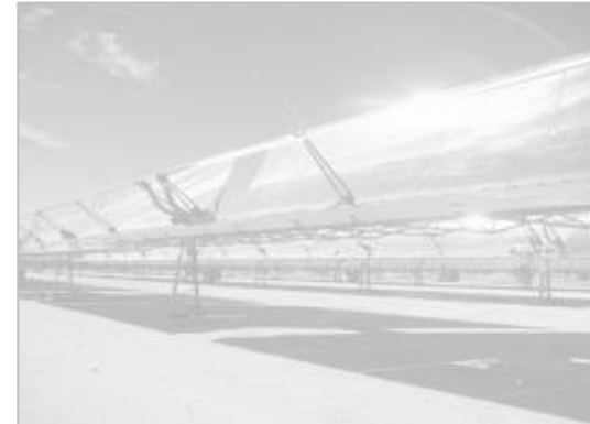
Concentrated Solar Power
