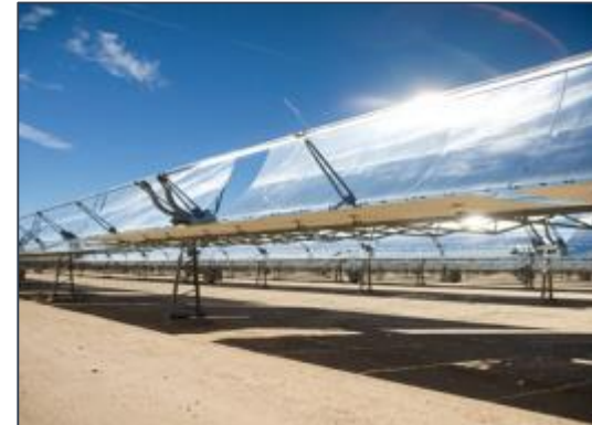
Concentrated Solar Power
