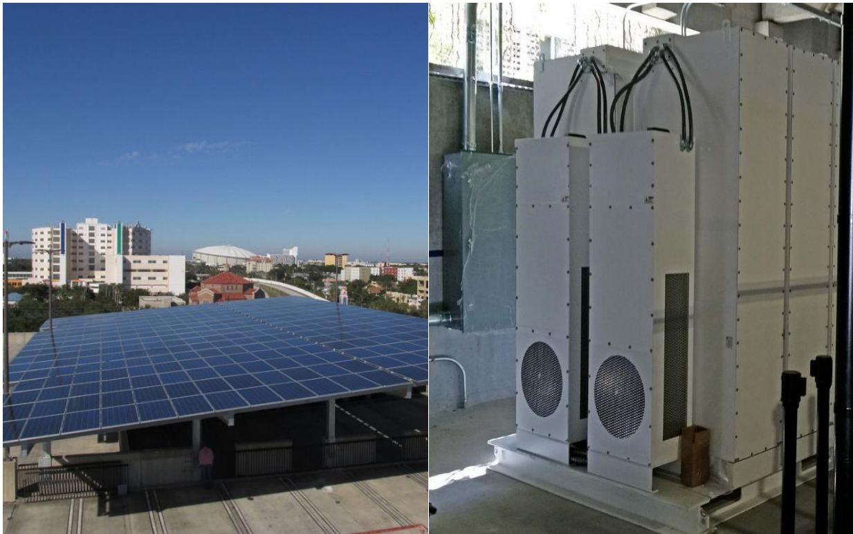
Figure 14. Solar and Energy Storage system at the University of South Florida 45
