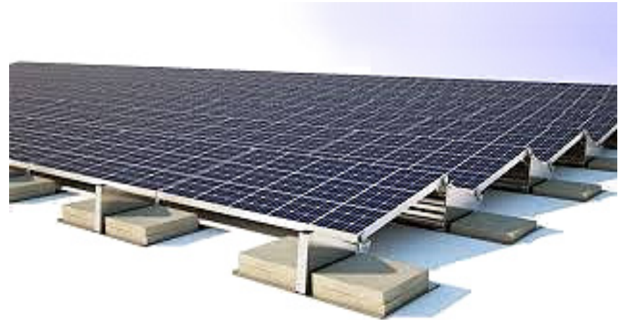
Another ballasted array. This one uses aluminum plates for the ballast blocks.
